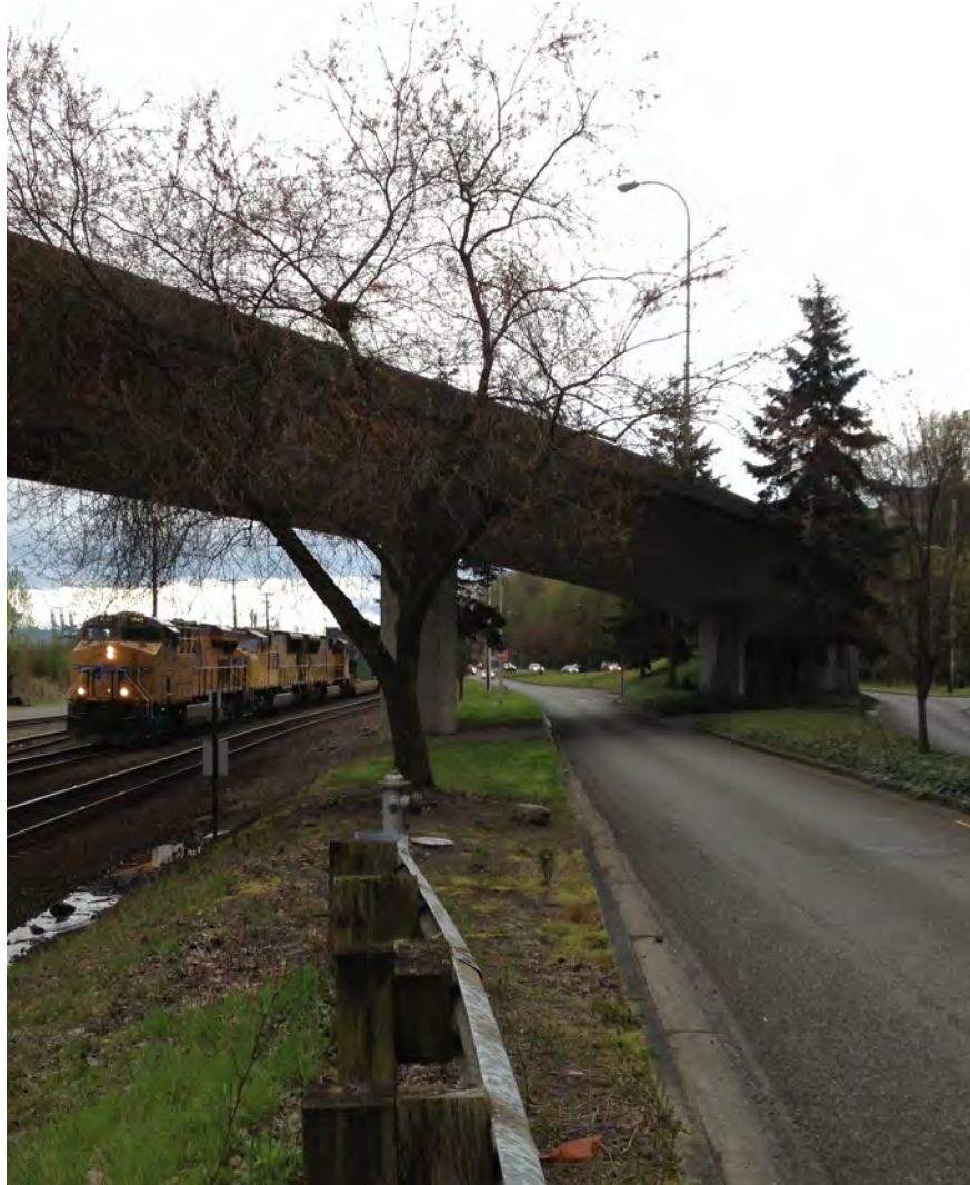
Existing Conditions at site of proposed two-step crossing of N. 30th St.
