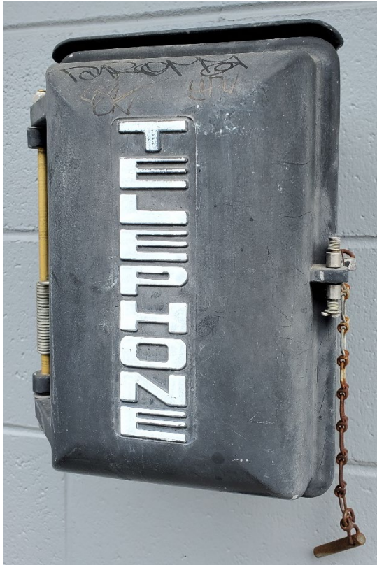
Rear Door Intercom
