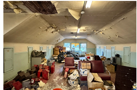
Figure 130. EMB's attic storage area is in poor condition
