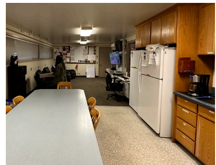
Figure 92. Station 9's dining area has poor finishes and ventilation
