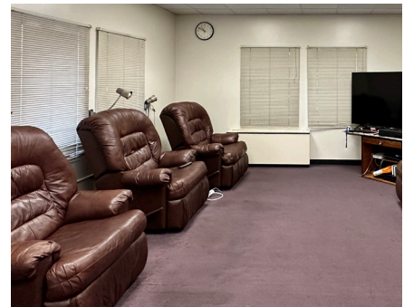
Figure 38. Carpet in Station 1's day room is dated and stained
