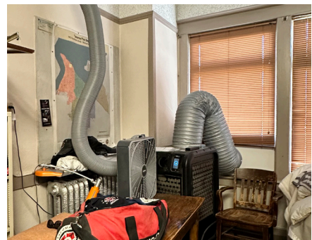
Figure 75. HVAC system in Station 11 dormitory
