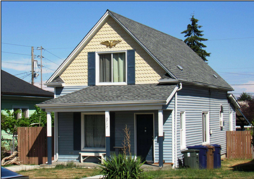
Figure 9. 3717 South Yakima Avenue has had a number of modern alterations, including the introduction of vinyl siding, which is an incompatible material for a building dating to the start of the twentieth century.
