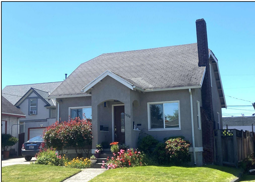
Figure 8. 3828 South Park Avenue has had all of its visible windows and doors replaced.
