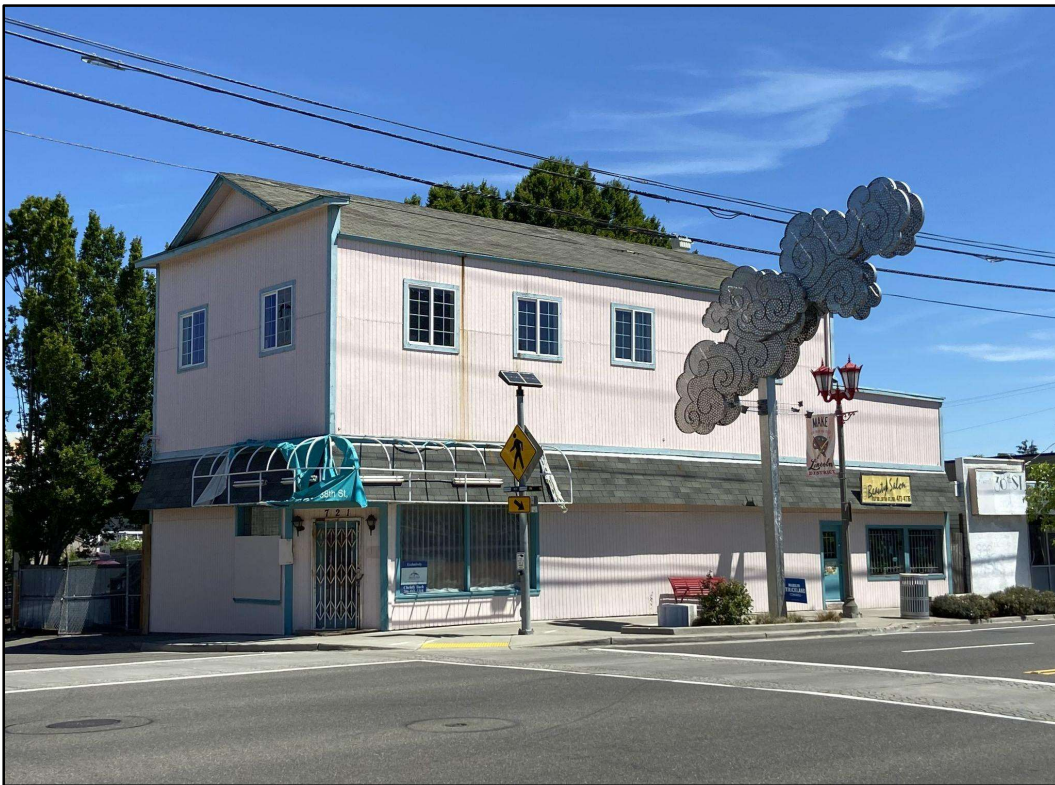
Figure 10. 717-723 South Yakima Avenue's clapboard siding was once a character-defining feature of the building. Now it is clad in T-1-11.
