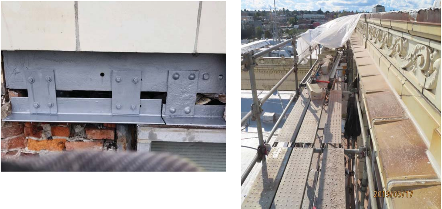
IMAGE 14. During: steel lintel repair detail (above left) and skyward facing joint sealant renewal (above right).
