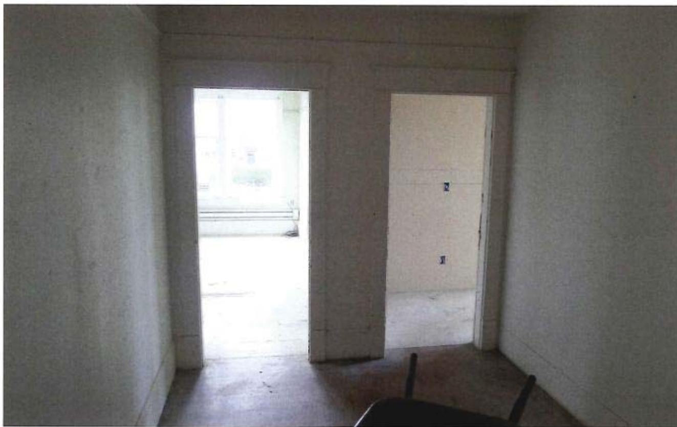
Interior, upper floor, looking west from hallway at entries to 2 units, SW and NW. March 2017.
