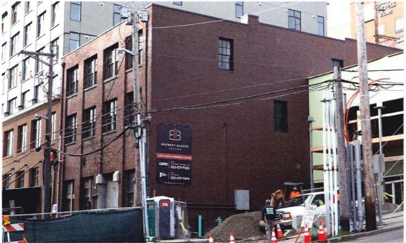
Northwest corner and north facade after work, September 2019. Note restoration of 2nd floor window.
