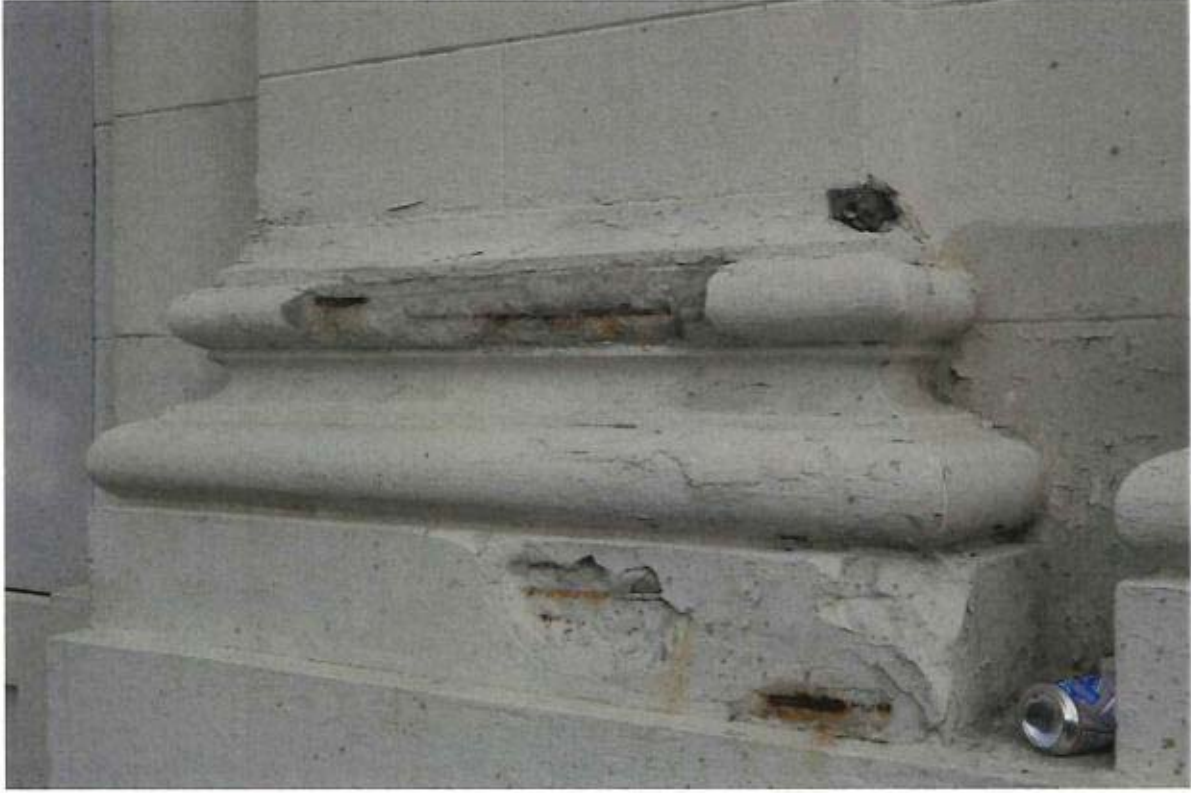
West facade detail, showing typical concrete deterioration on exterior. 2016.
