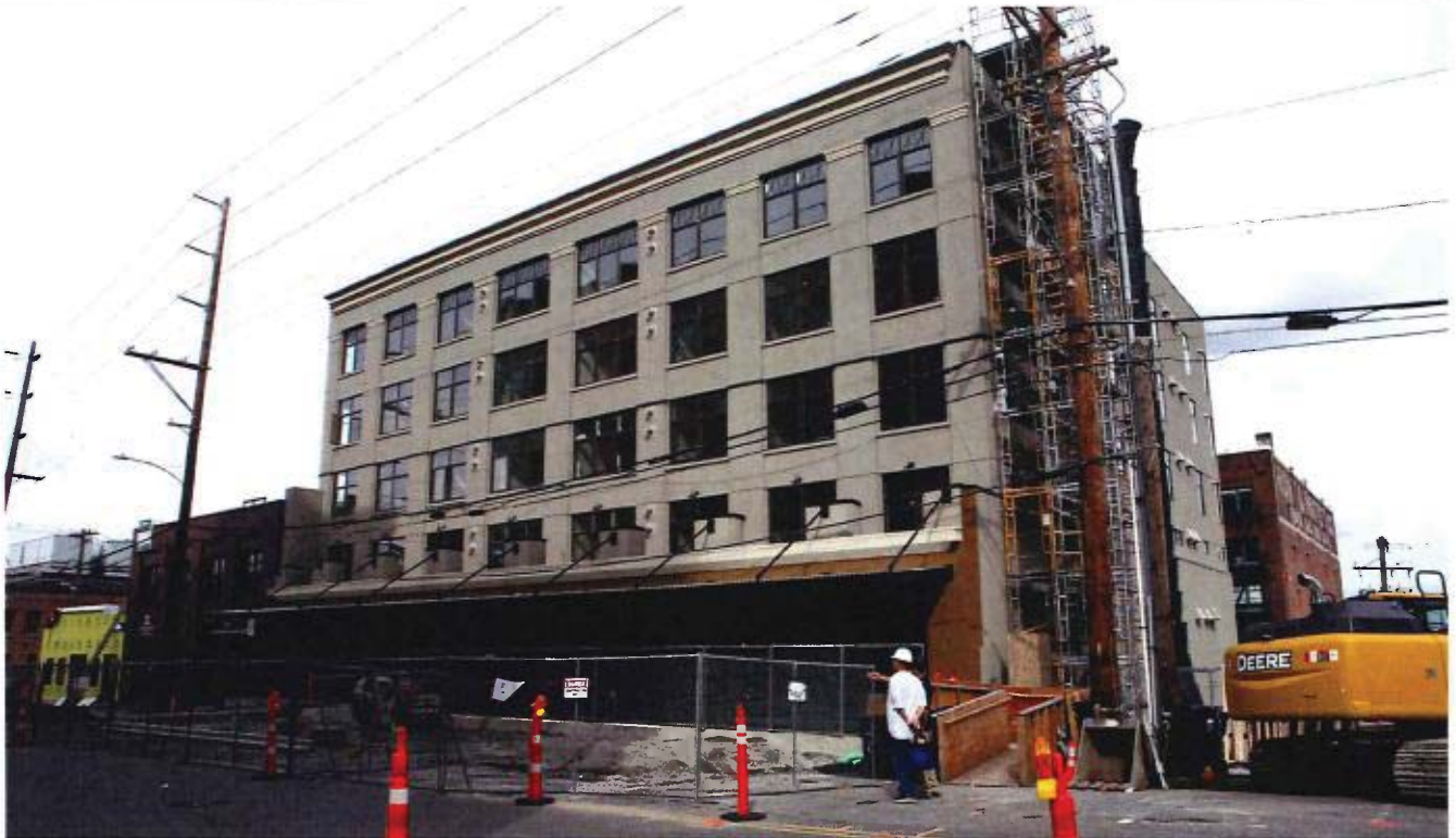
Southwest corner in September 2019, showing completed work. New upper stories not counted in project costs.
