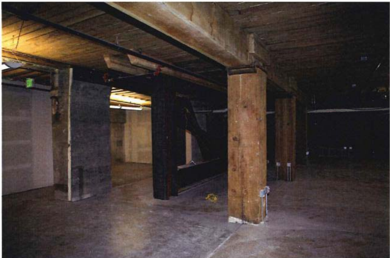
1st floor, typical open space with large wood posts, added steel and concrete reinforcement. September 2019.
