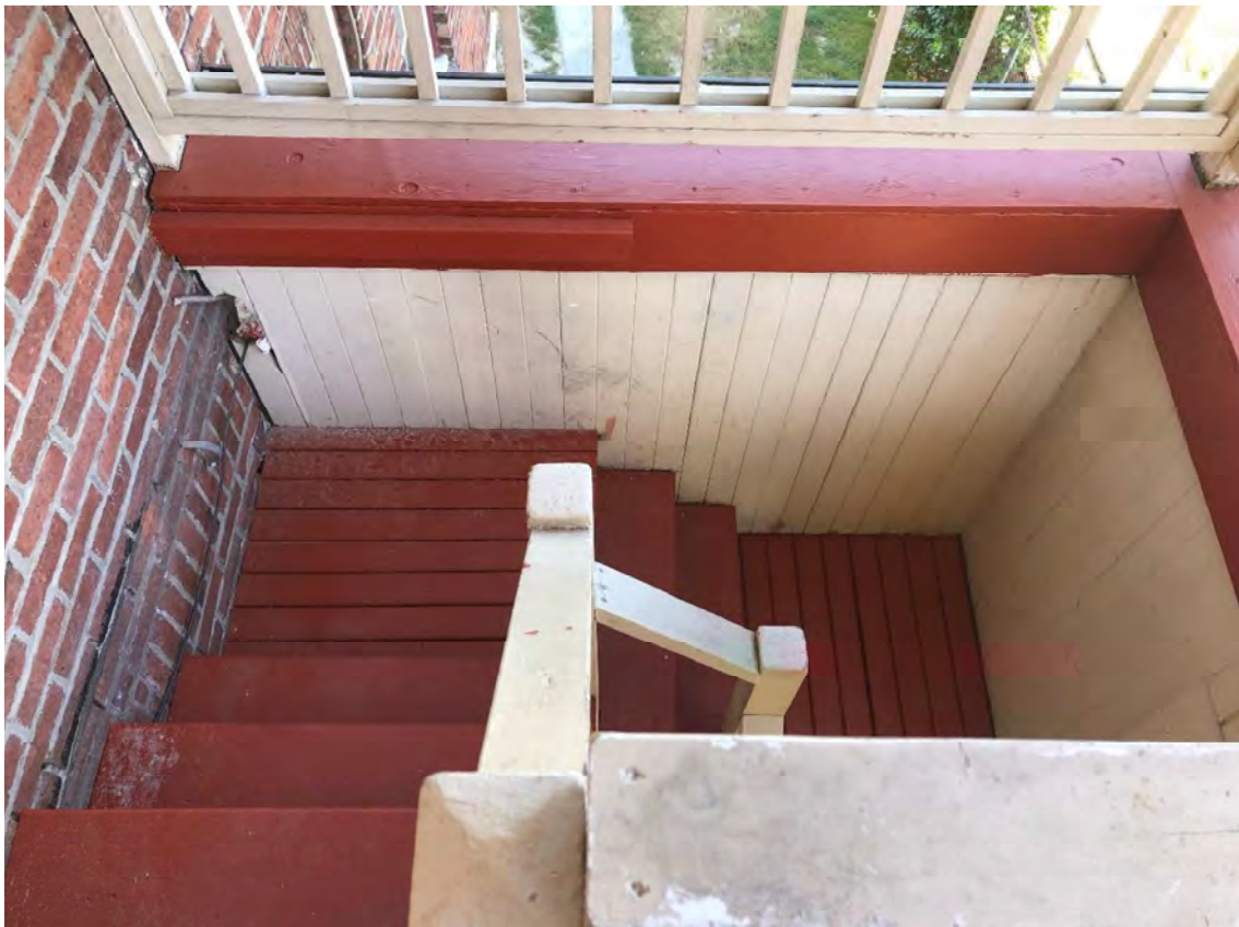
Fig. 25B (After). Rear egress porch, stair down from Second Floor landing, looking north, August 2020. Source: Stephen Day Architecture.
