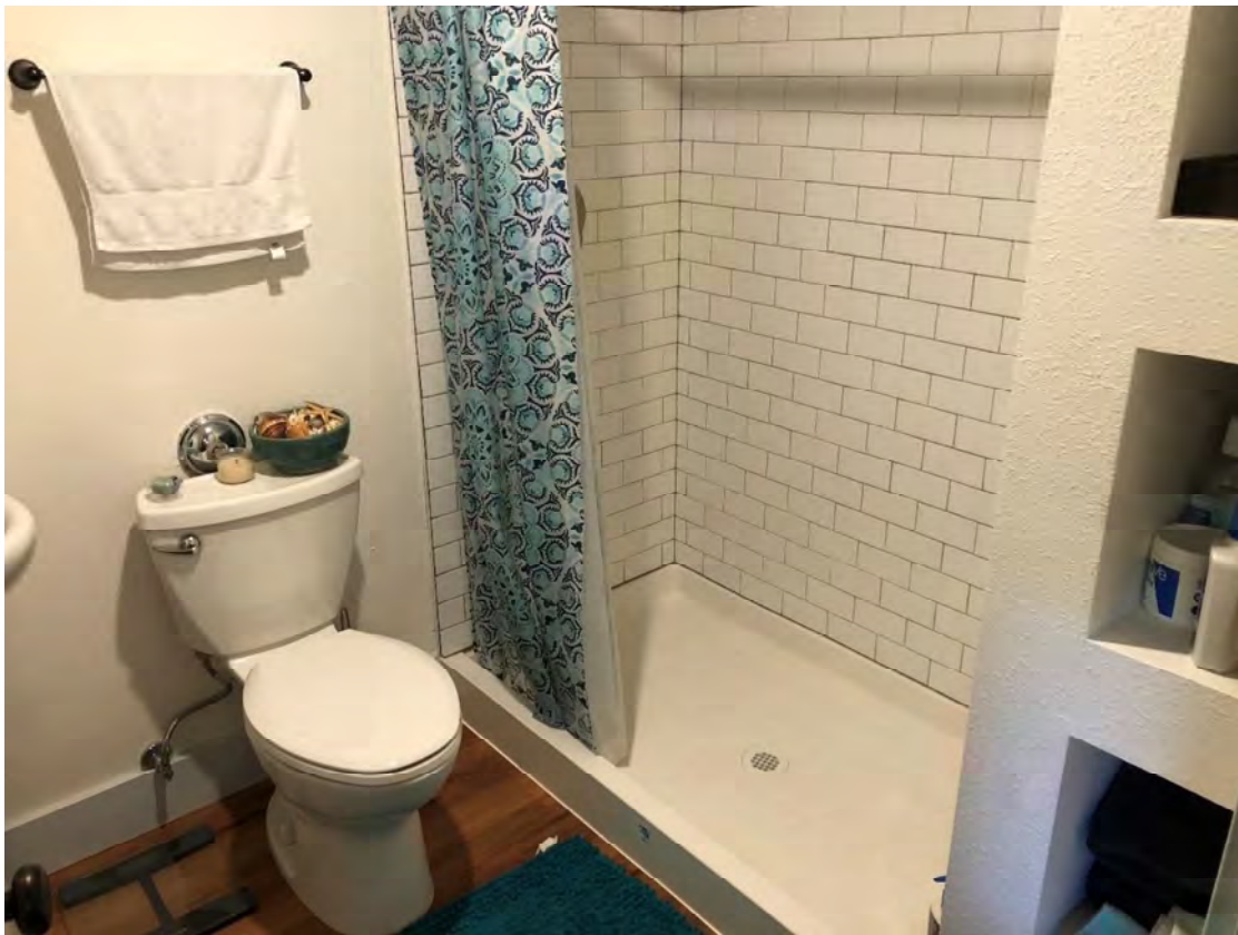
Fig. 34D (After). Newton Apartments, former Basement Unit 18, looking southeast in bathroom. August 2020. Source: Stephen Day Architecture.
