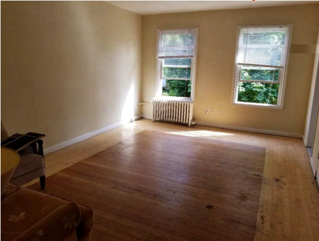
Fig.42. Newton Apartments, Typical Second Floor unit, Unit 12, original oak/fir floor, looking southeast, 2018. Source: Owner.
