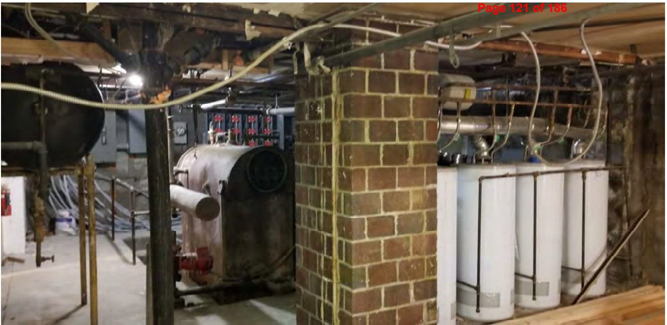
Fig. 32. Newton Apartments, boiler room and utilities space. Looking southeast, 2018. Source: Owner.
