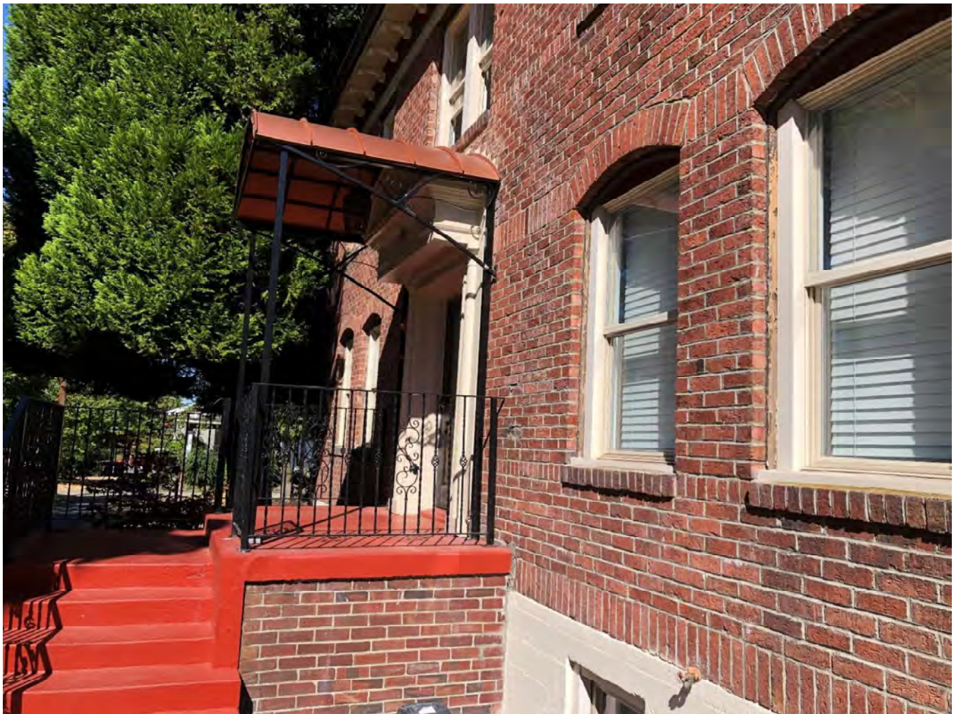
Fig. 21 (After). Newton Apartments front porch, looking north, with new awning and support. August 2020. Source: Stephen Day Architecture.
