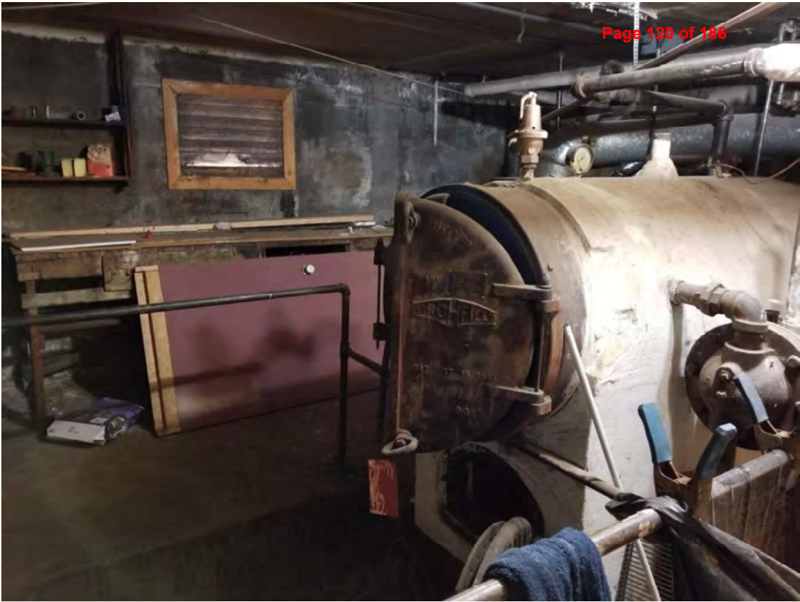
Fig. 31. Newton Apartments, boiler room and utilities space. Looking southeast, 2018. Source: Owner.
