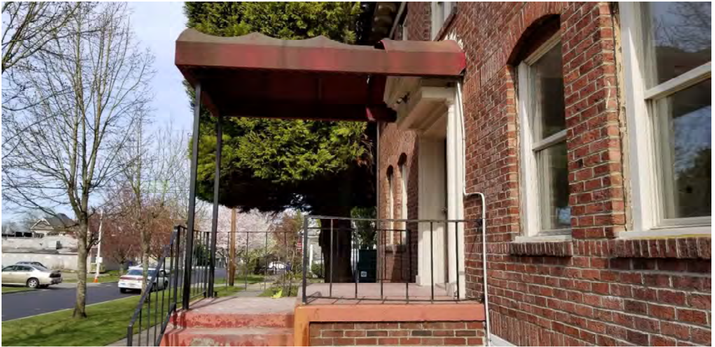
Fig. 21. Newton Apartments front porch, looking north, 2018, prior to removal of damaged awning and support. Source: Owner.
