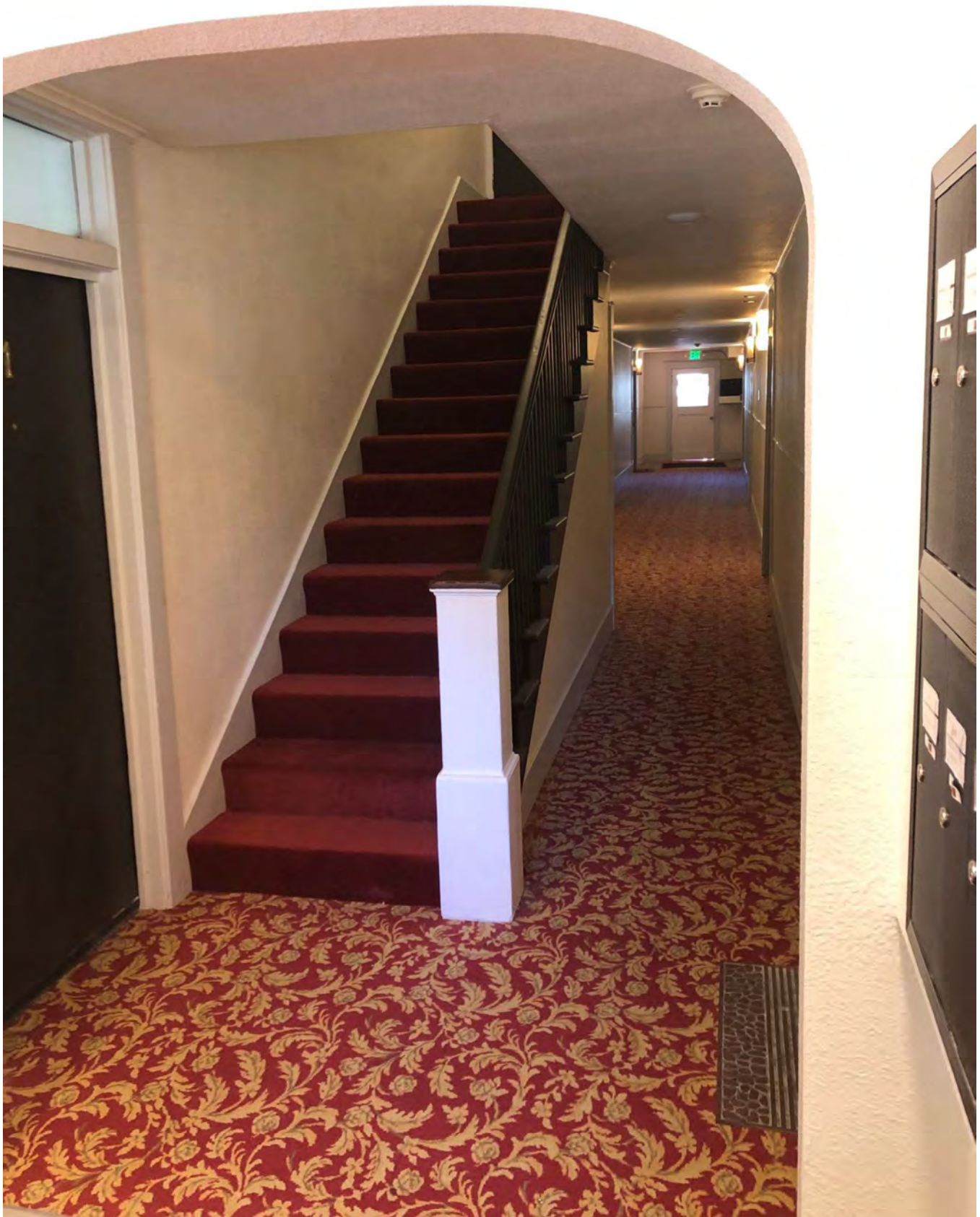
Fig. 26 (After). Newton Apartments, entry foyer and stair from First Floor to Second Floor, looking east. Carpet at stair and corridor replaced, balustrade, top rail and newel post repaired. August 2020. Source: Stephen Day Architecture.
