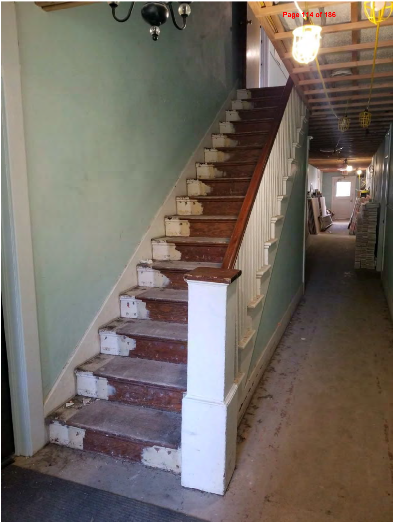
Fig. 26. Newton Apartments, entry foyer and stair from First Floor to Second Floor, looking east. Note carpet at stair and corridor removed, ceiling plaster at corridor removed as electrical rewiring started. November 2019. Source: Owner.
