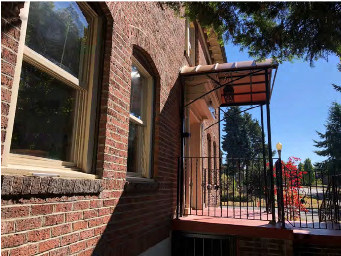
Fig. 16 (After). Newton Apartments, north façade, egress from Basement (below front porch), looking south. August 2020. Source: Stephen Day Architecture.
