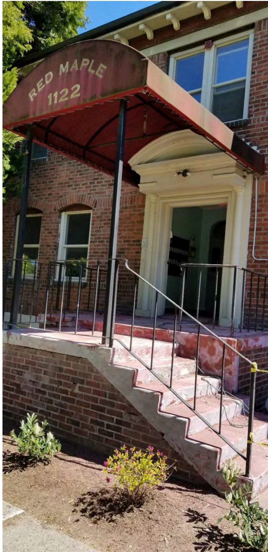
Fig. 22. Newton Apartments front porch, looking northeast, 2018, prior to removal of damaged awning and support. Source: Owner.
