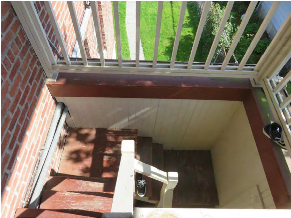
Fig. 25B. Rear egress porch, stair down from Second Floor landing, looking north, 2018. Source: Owner.
