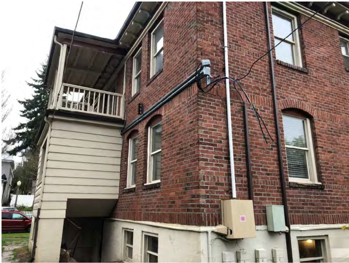
Fig. 10. Newton Apartments, porch at east façade, looking south. December 2019. Source: Stephen Day Architecture.
