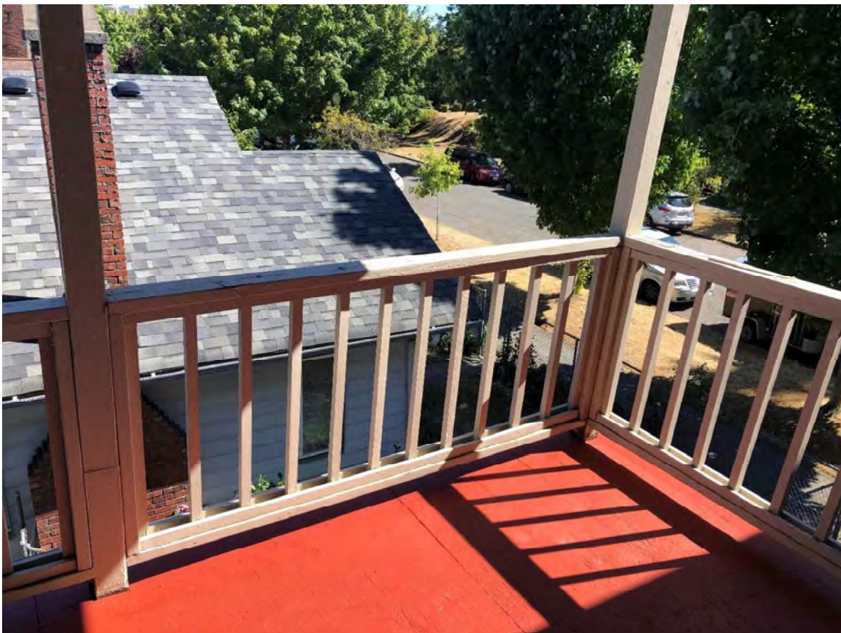
Fig. 25A (After). Rear egress porch, at Second Floor landing, looking southeast, August 2020. Source: Stephen Day Architecture.
