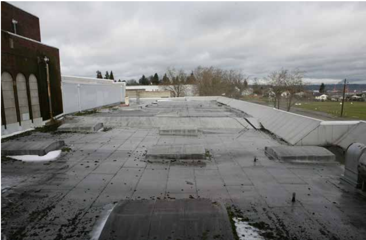
CP64. Looking north over roof of east side of original building. (Taken from Classroom 206/Band Room)
