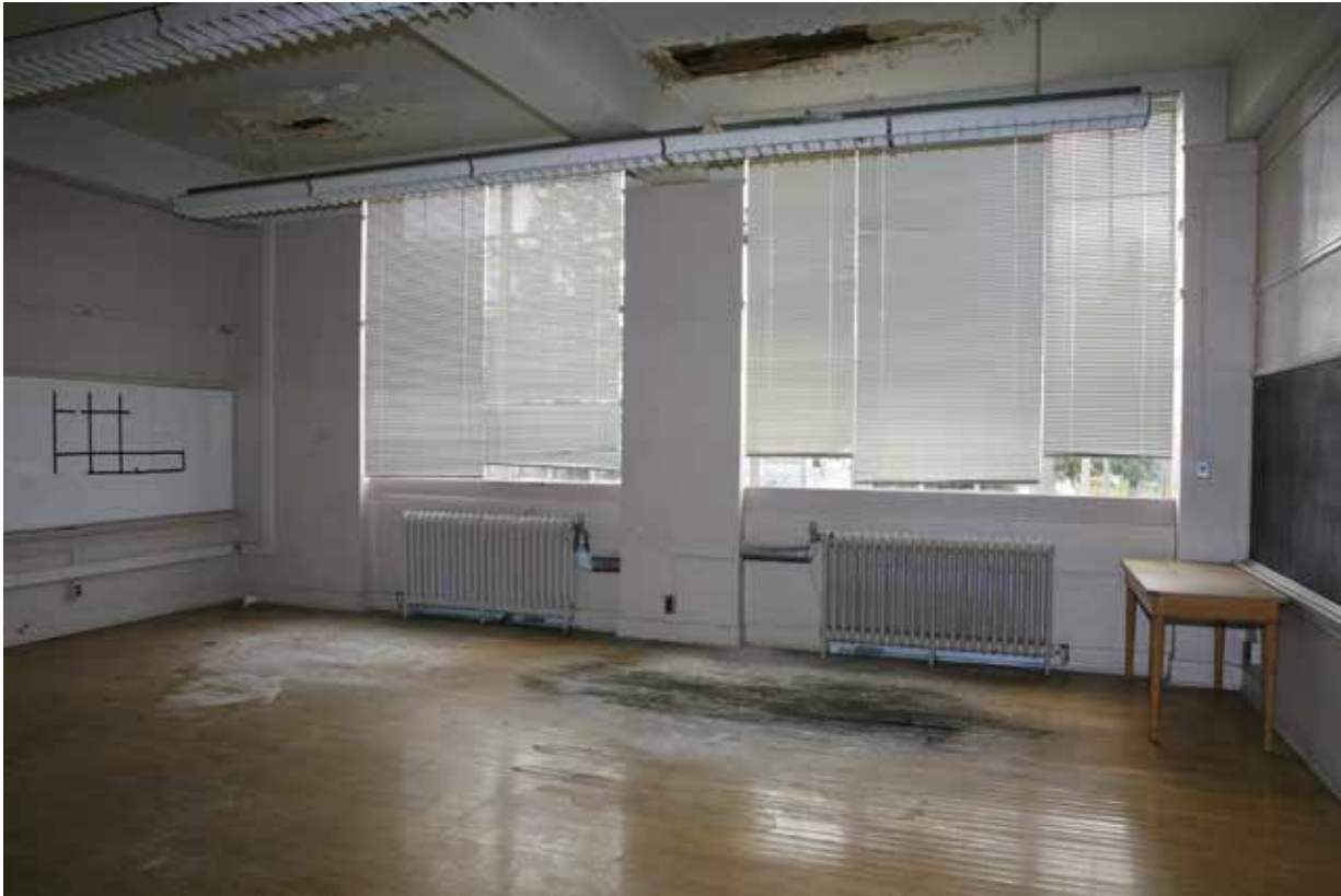
CP63. 2nd floor, Classroom 204, looking SE. Note wood floor, blackboard. Water damage to ceiling and floor.
