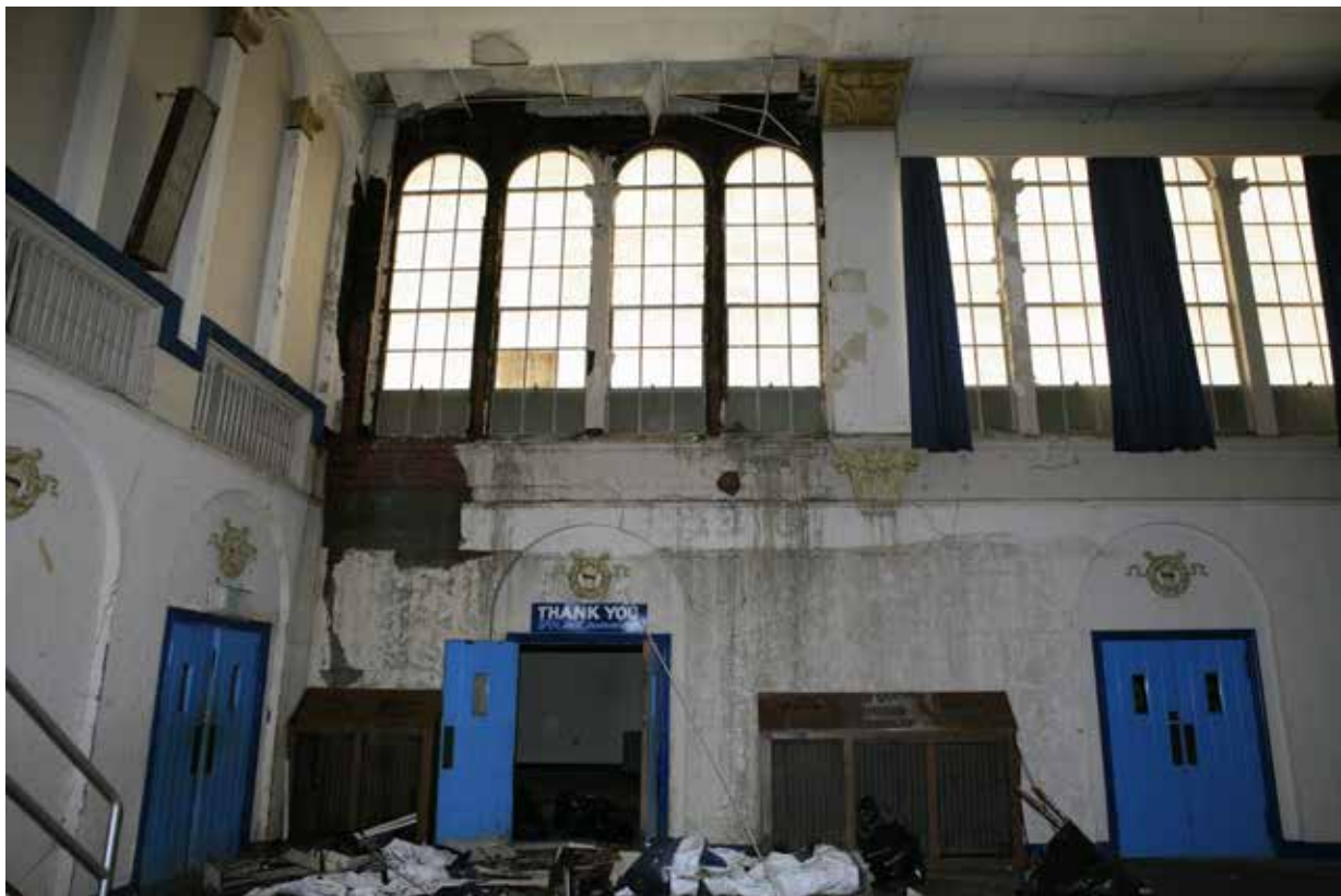
CP38. Auditorium, NE corner, looking east. Note water damage from roof leak.
