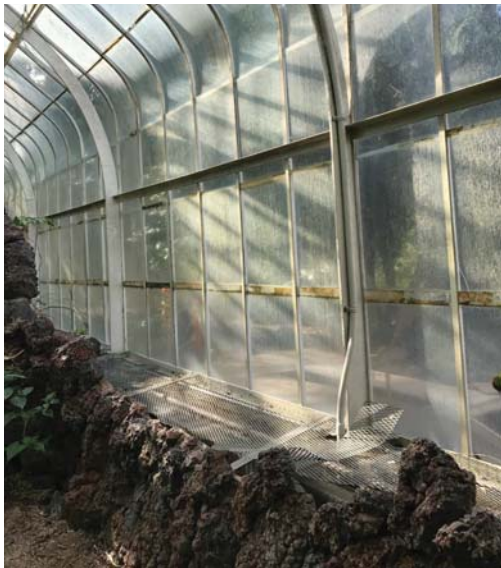
EXISTING SLAG WALL (protecting fin tubes)
