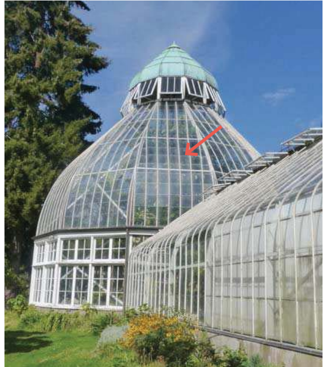
Today, joints are even at the dome.
