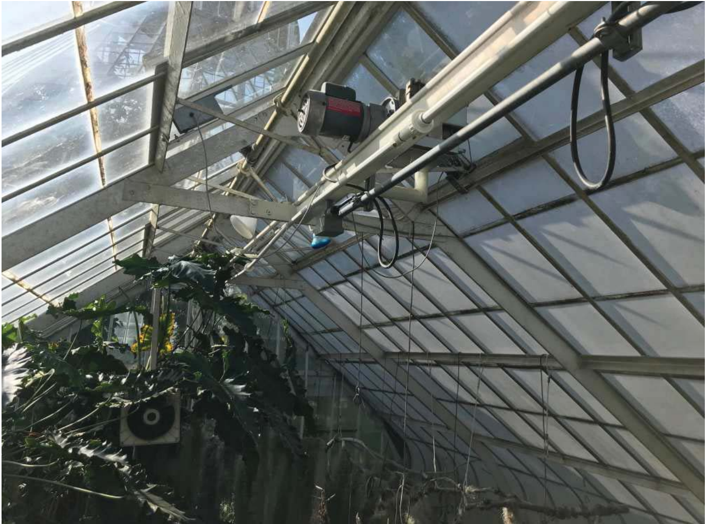
EXISTING SYSTEMS AT THE PEAK OF THE GABLE WINGS (This proposal aims to simplify these systems)
