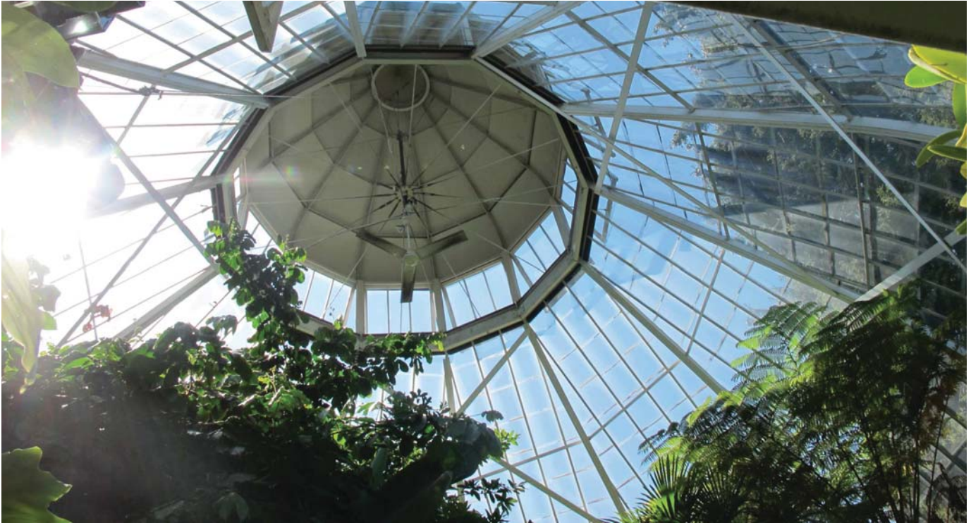
FLAT PLATE CROSS BRACING AND FAN AT THE ROTUNDA (Added as part of the 2003 renovation)
