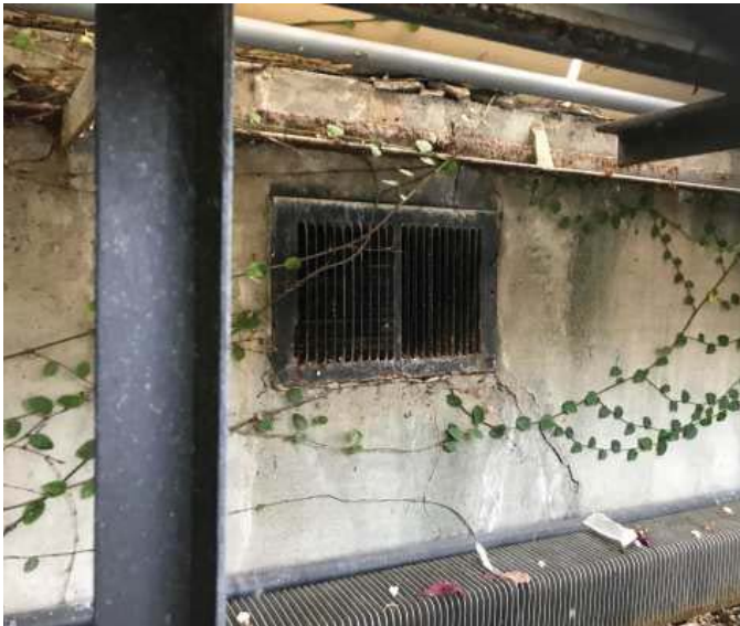
EXISTING INTAKE VENT (The exterior of these vents were patched as part of the 2003 renovation)
