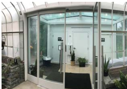
CUSTOM METAL FABRICATED THRESHOLD FROM STEEL PLATE, AND ALUMINUM FRAMED GLASS ENTRANCE DOOR, WHITE (TO MATCH RESTROOM ADDITION)
