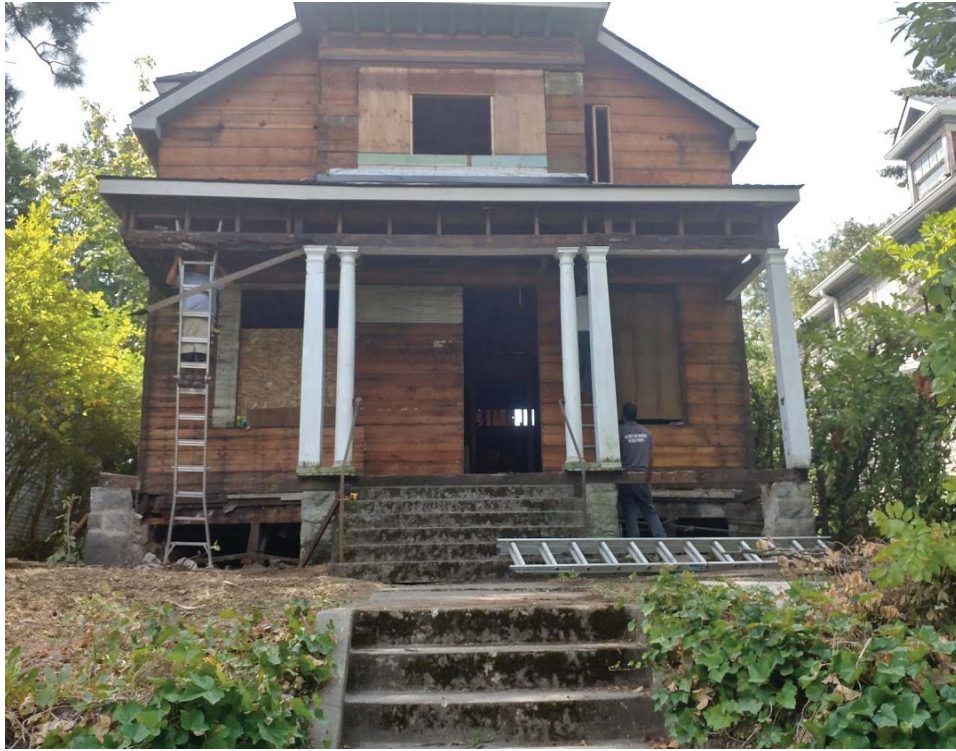
Exploratory demolition of the front porch showed extensive rot.
