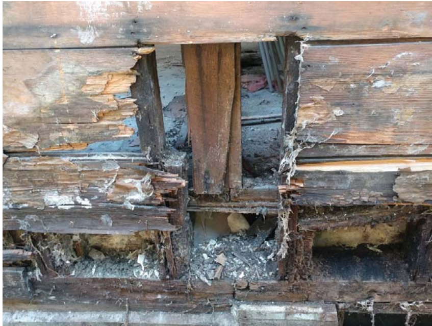
Areas of rot revealed after removal of asphalt siding
