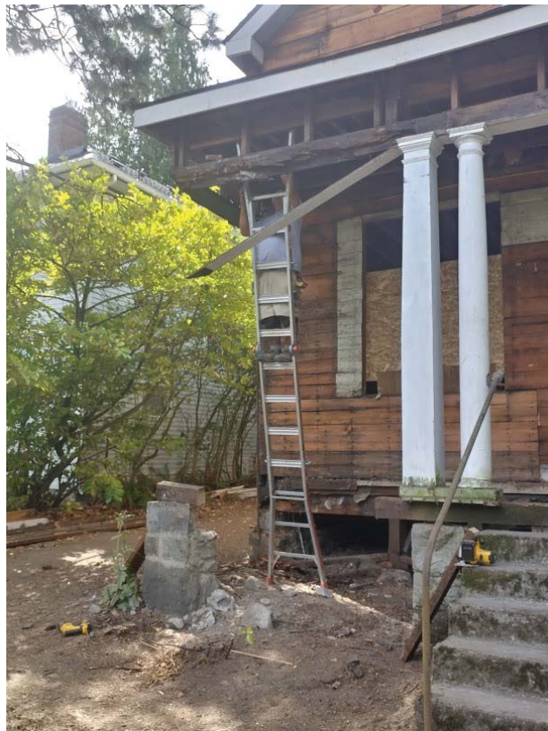
Additional photo showing rot in the head beam
