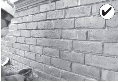
Re-point mortar joints where there is evidence of deterioration. This shall match the historic design.
