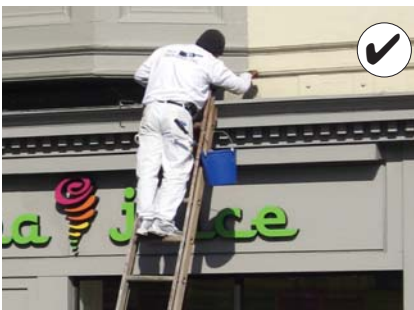
Repair deteriorated building materials, when needed.
