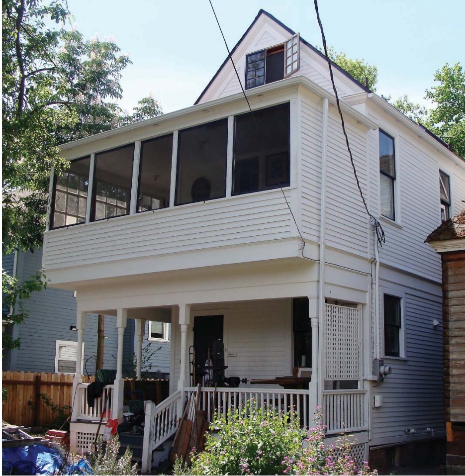
Figure 5. East (rear) and portion of north façade. Note the turned porch posts and the glass panes on the south side of the sleeping porch.
